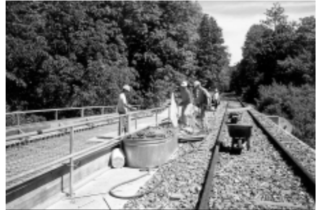
A construction crew works on the York County Heritage Rail-Trail. Photo: Gaven Loose
