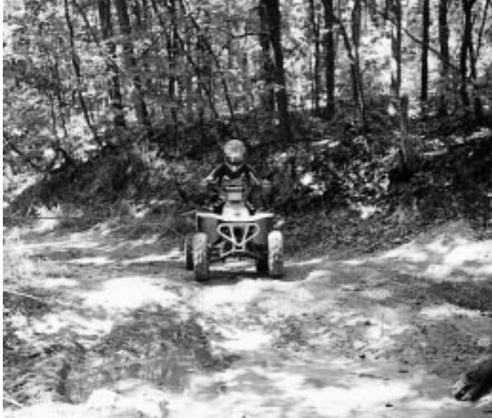
This water-saturated trail tread indicates improper location, improper design or both. This trail should have had an interceptor ditch located 10 feet uphill (See interceptor ditches).
