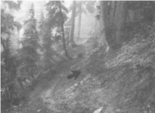
"Full Bench" construction is often required on steep slopes or weak soils. Note how this trail has slipped downhill.
