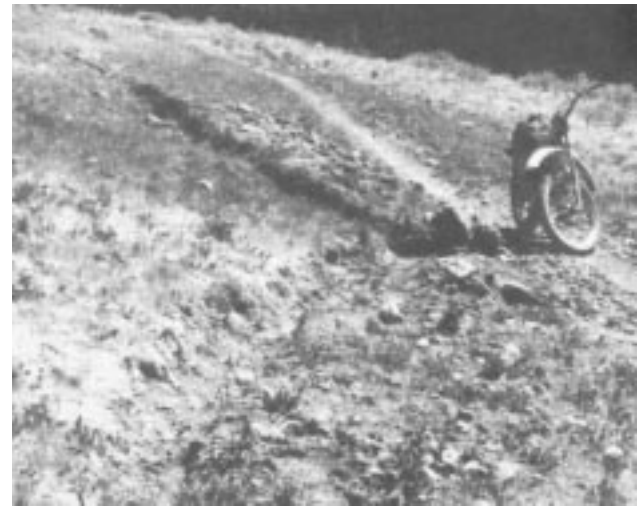
This properly constructed collector ditch intercepts ground water before it can saturate the trail tread.
