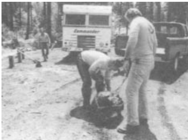
Organized volunteer groups can play an important role in maintaining trails and other related facilities. Here, volunteers help to construct a trail staging area and campsite.
