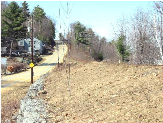
This height of this gabion wall would be increased to support a trail along the west side of the railroad (see Section G, Sheet 19).
