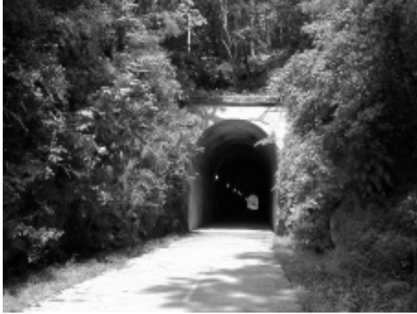
The Brushy Mountain Tunnel on the Silver Comet Trail in Paulding County, Ga., provides an excellent example of both an attractive portal and long sight lines. Credit: PATH Foundation.
