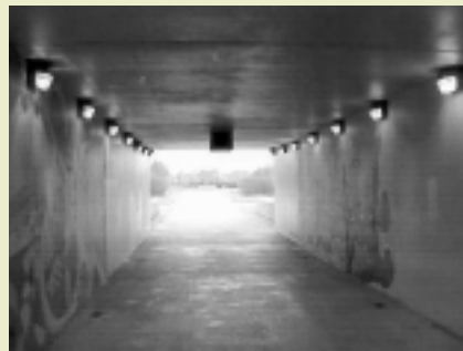
The I-90 tunnel in Washington utilizes two security cameras, one of which is visible on the ceiling of the tunnel. Credit: Washington State Department of Transportation.
