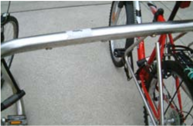
Choosing inappropriate materials will compromise security. Welded sections of this stainless steel rack have been broken off by vandals or thieves.
