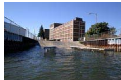
Piers at County Boat Ramp are in bad condition (Photo: FMR)
